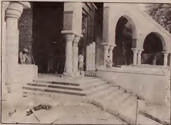
The Palmer Museum of Art at University Park is beginning to take shape. Scaffolding, erected as part of the $5.6 million renovation and addition project, has been removed and workers will soon begin to install the plaza area that will grace the front entrance. The museum should reopen to the public in June of 1993.
